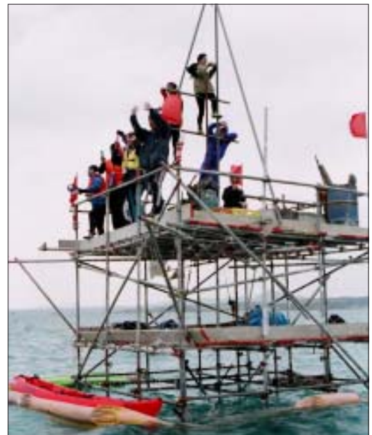
The test boring points have been occupied daily from sunrise until sunset
